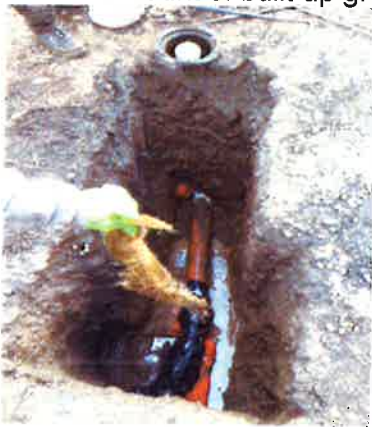
This is a root ball taken from a sewer lateral on 3 rd .
