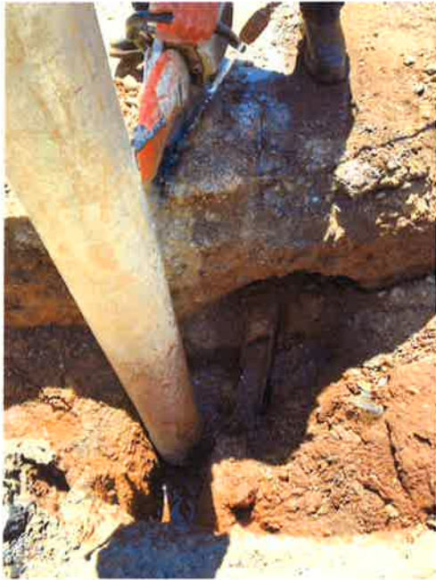
Broken 4” water main on Lakeview
