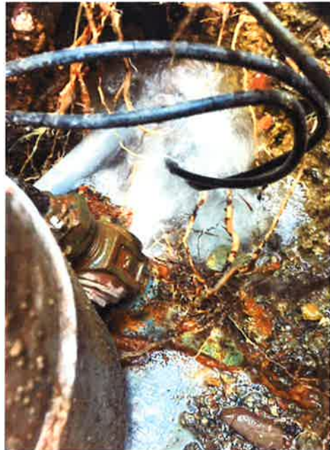
Leaking saddle on Anchor
