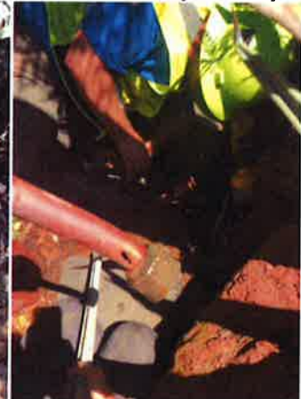
The line that pulled apart.
