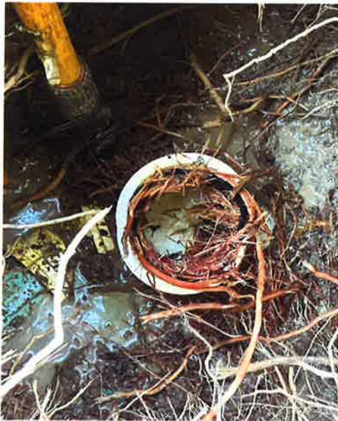
Sewer lateral full of roots
