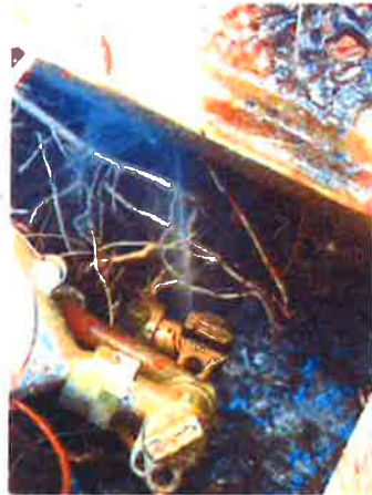
Leaking curb-stop & gasket
